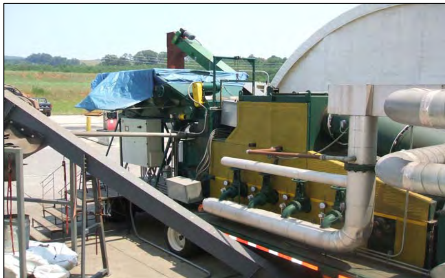
Photo #2: Ecoremedy™ gasifier installed and operating
